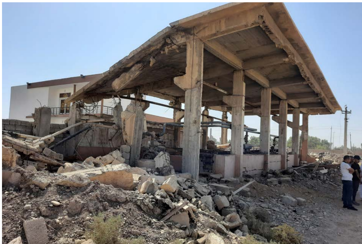
Figure 9: One of the ice factories which got damaged in the June 2015 airstrike, September 2021. PAX/Saba Azeem.
