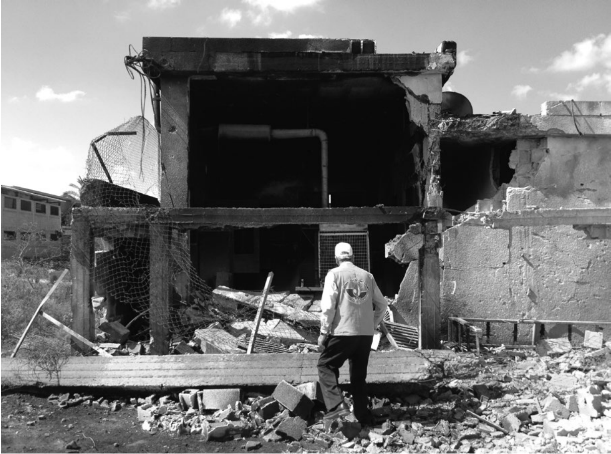
An engineer from the Coastal Municipalities Water Utility inspects a damaged sewage pumping station in Beit Hanoun, a high density urban area close to Gaza City.
